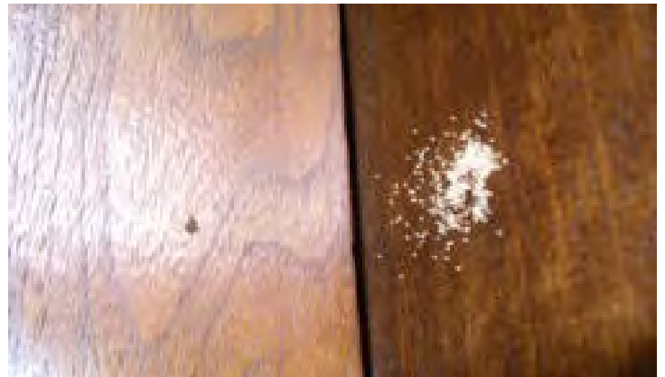
Drywood termite fecal pellets.
